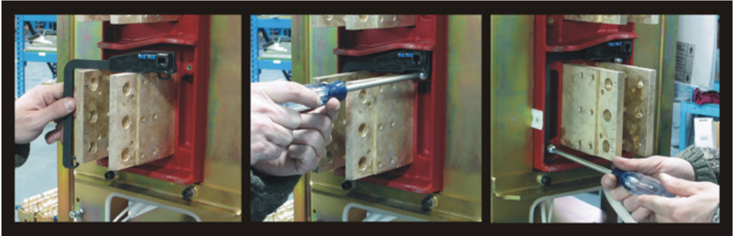
Replace with single new sensor and new hardware to lower bus.
