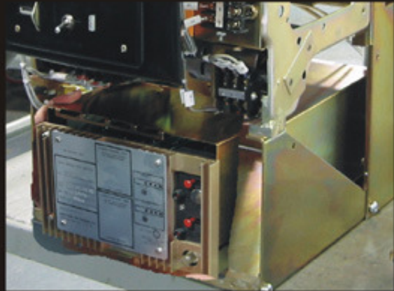
FBK circuit breaker with ABB trip unit to be replaced.
